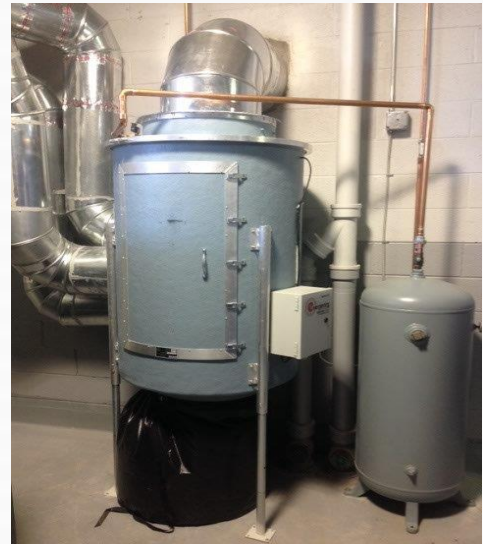
Fire-Retardant Fiberglass Filter w/ Dryer Ducts
